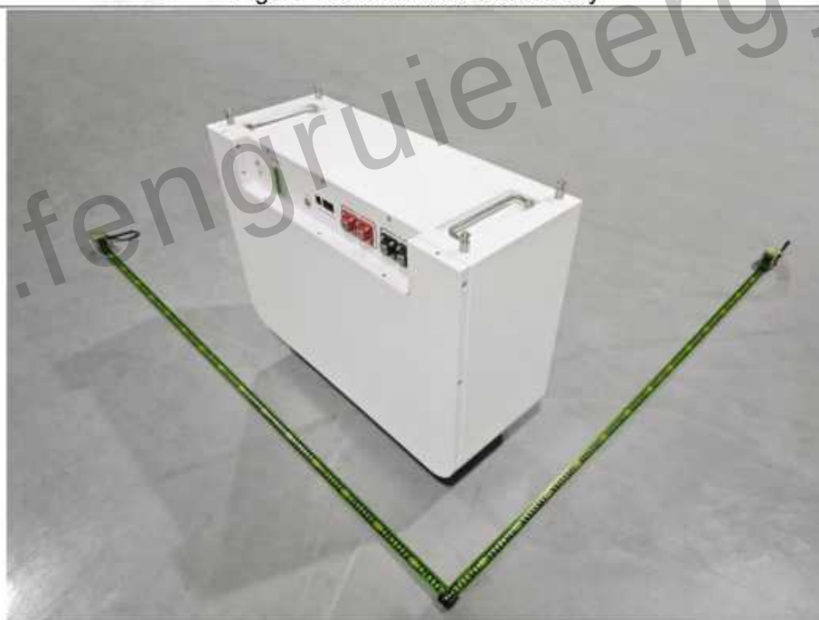
Figure 2 Overall view 2 of Battery
